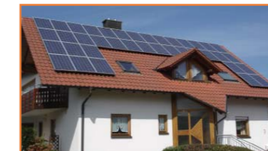
Off-grid home solar system
